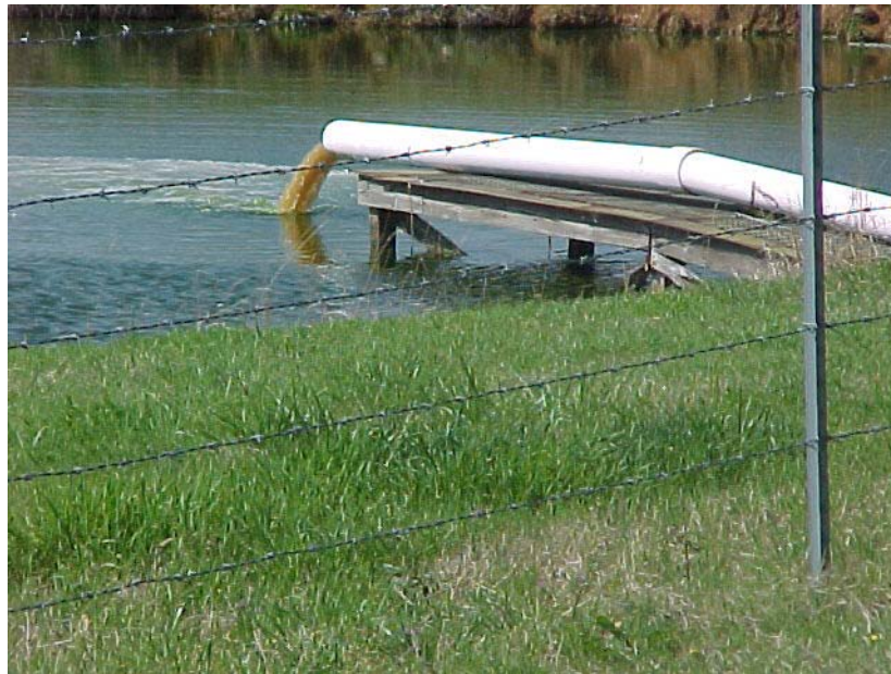
Figure 3.4. Flushing of wastewater to the lagoon
