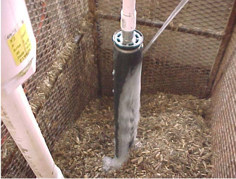
Figure 3.10. Membrane diffuser installed in the bioreactor
